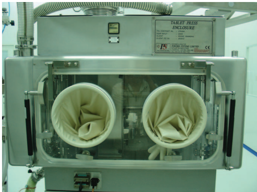
Shanghai Roche installed an isolator to reduce API concentrations to 0.01 \text{ mg}/\text{m}^3 , protecting the operators.
